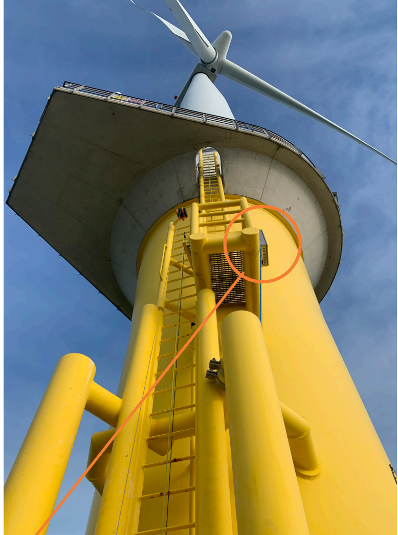
Figure 3: PLC Enclosure, London Array Wind Farm (Kent, UK)
